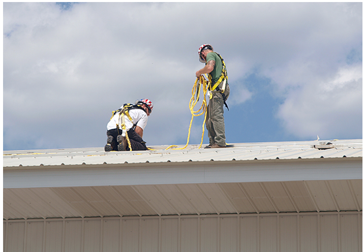
Installers from the Radiant Store in Troy, NY get a roof ready for solar thermal. (Photo courtesy: NYSERDA)
